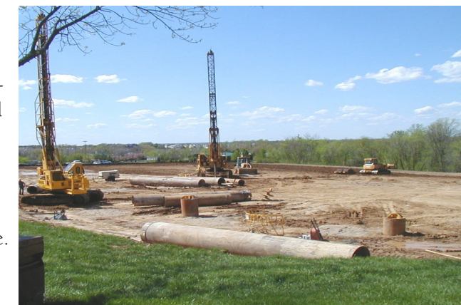
Construction is underway in the 16000 block of Chesterfield Parkway West on Central Park Square I, the latest office building at Chesterfield Village.
